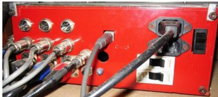
Figure 13. Small Mill Control Cabinet front panel.
